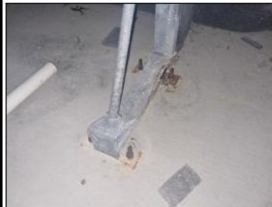
Photo 4 – Corrosion to base plates and bolted connections
