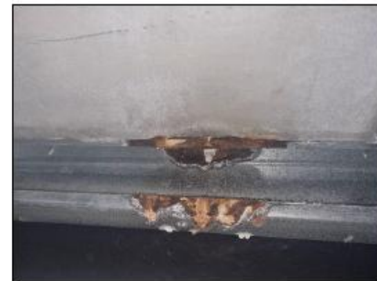
Photo 3 – Corrosion to 'Rondo' channel sections
