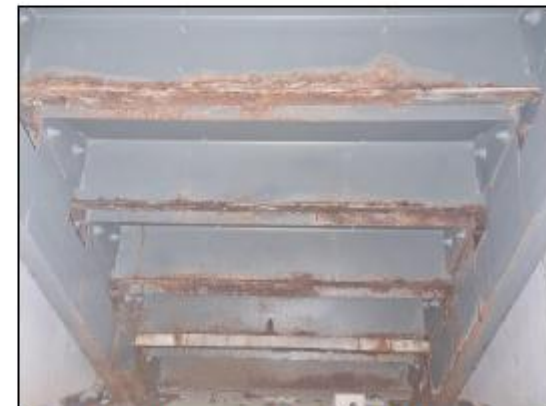
Photo 5 – Corrosion to pool access staircase (treads, stringers & brackets)
